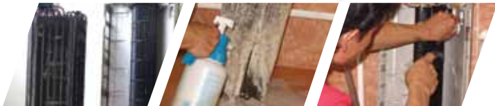
Before Chemical Wash
