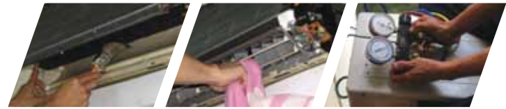
Brush & check cooling coil
